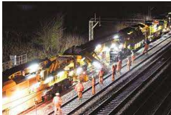
Fig. The West Coast Main Line requires regular night time maintenance usually closing two tracks. We only have two!
